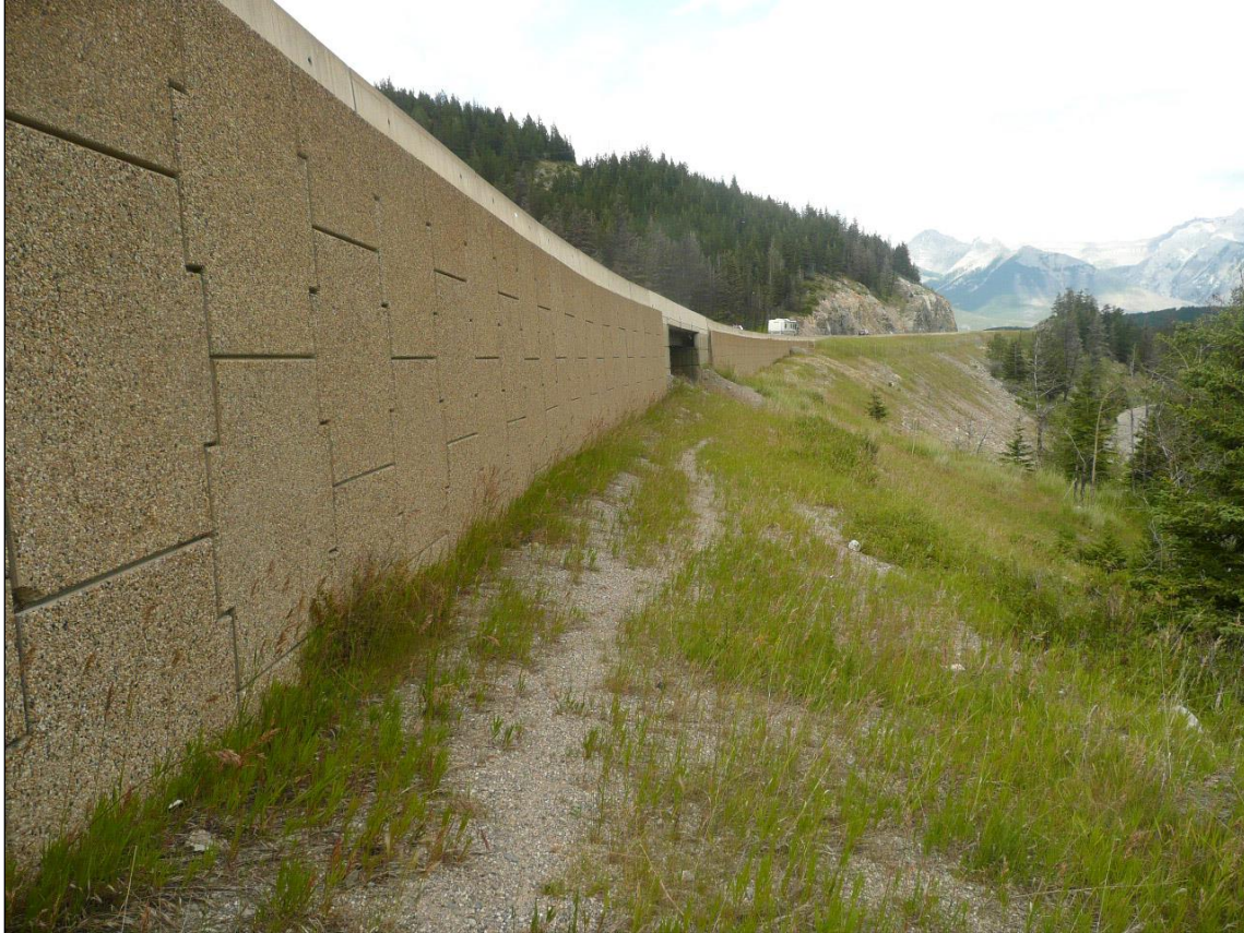
Mechanically stabilized earth (MSE) wall serving as wildlife exclusion “fence” (Photo: Tony Clevenger).
