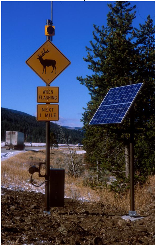
Animal detection system along Highway 191 in Yellowstone National Park, Montana (Photo: Marcel Huijser, WTI).
