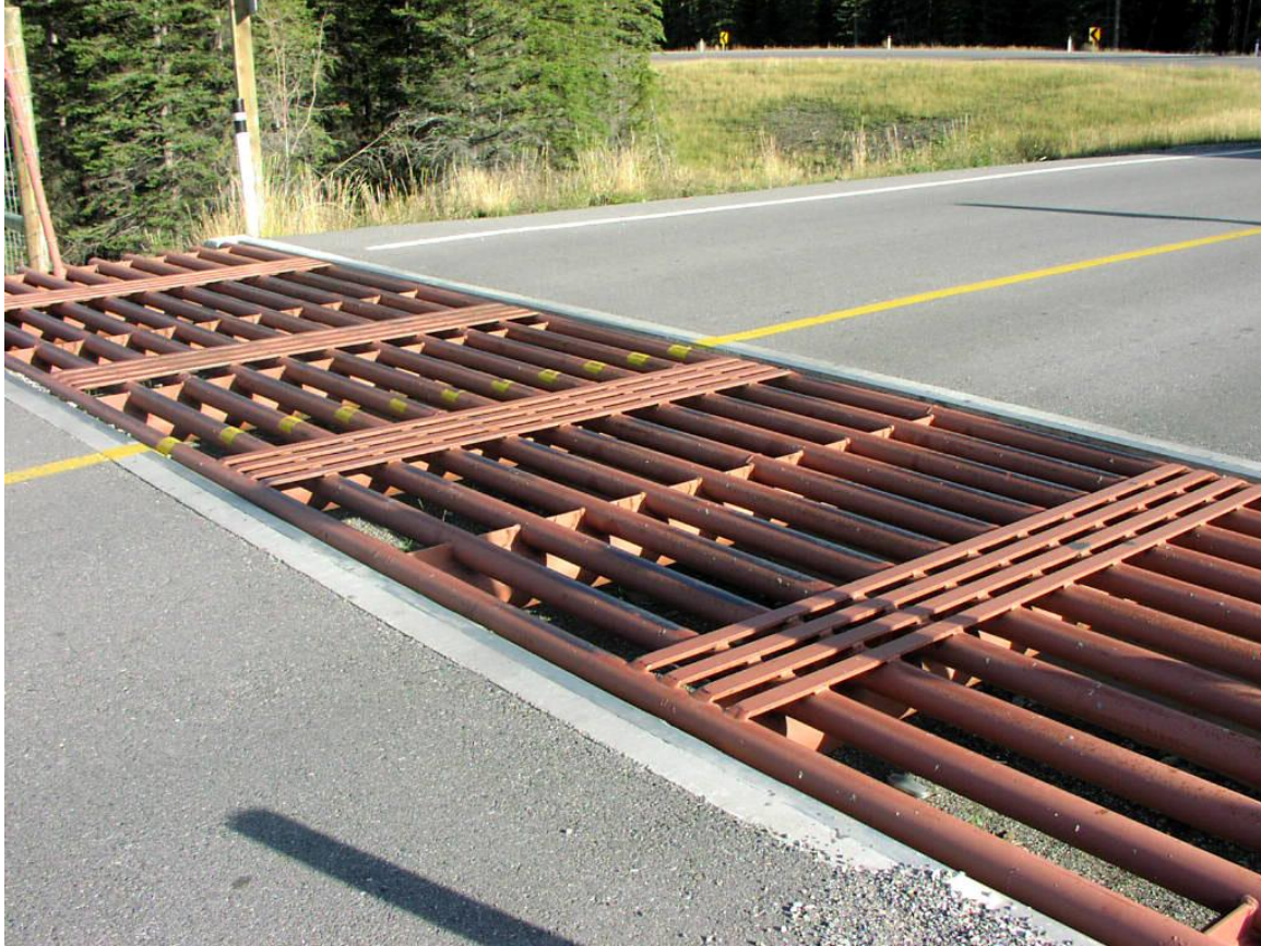
Cattle guard (Texas gate) in road (Photo: Tony Clevenger).
